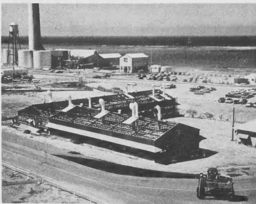
DISMANTLING IS underway on the old Zone 2 and C&LE office building, one of several on the surplus list at Lago. The EIG building is suffering the same fate.
